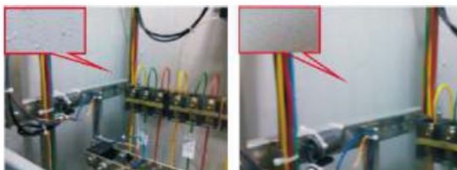
Before- Water on the wall
